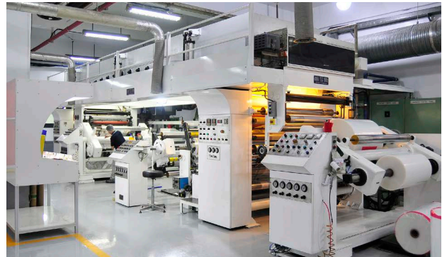
Converting Facility / Incheon, South Korea Prototype Development, Printing & Processing
